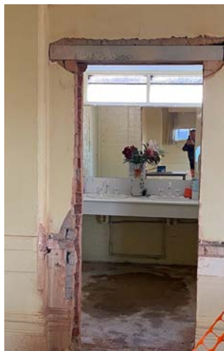
Works to create the new entry into the women's toilets from the main hall.
