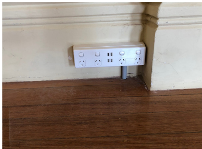
One of the eight new power and USB points in the hall.
