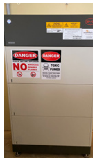
Our new battery, up on the balcony
