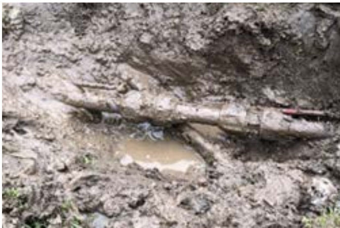
Leak on the 9th Fairway
